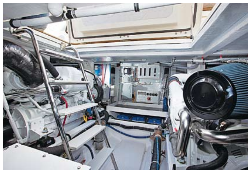
THE CUMMINS DIESELS WITH ZEUS DRIVES ARE BENEATH THE COCKPIT, ABAFT THE SALON. ALL SYSTEMS ARE EASY TO SERVICE.
